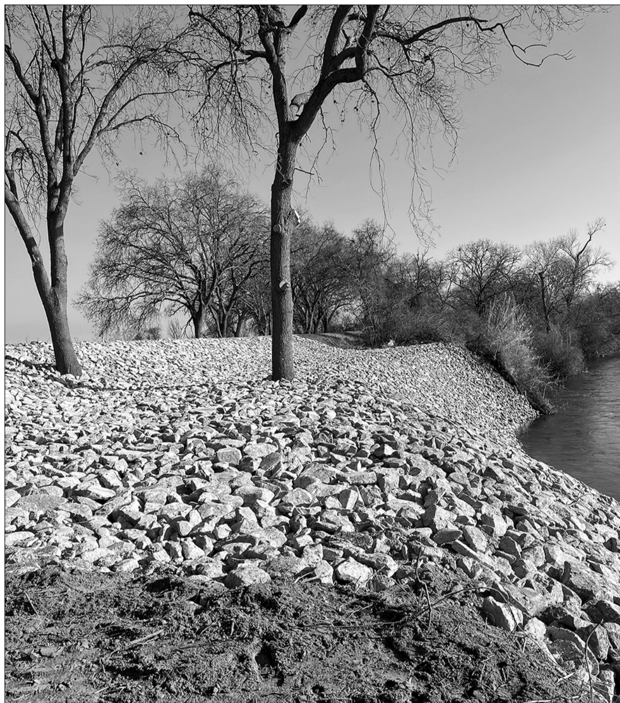
Completed emergency repairs to a levee south of the Folsom South Canal on the Sheldon side of the Cosumnes River are shown after heavy rains in early January. Courtesy photos
