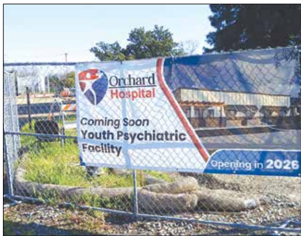
Site work is underway for Orchard Hospital's new youth psychiatric health facility, a project expected to expand behavioral health services in Butte County. Photo by Mickey Mrakuzic
