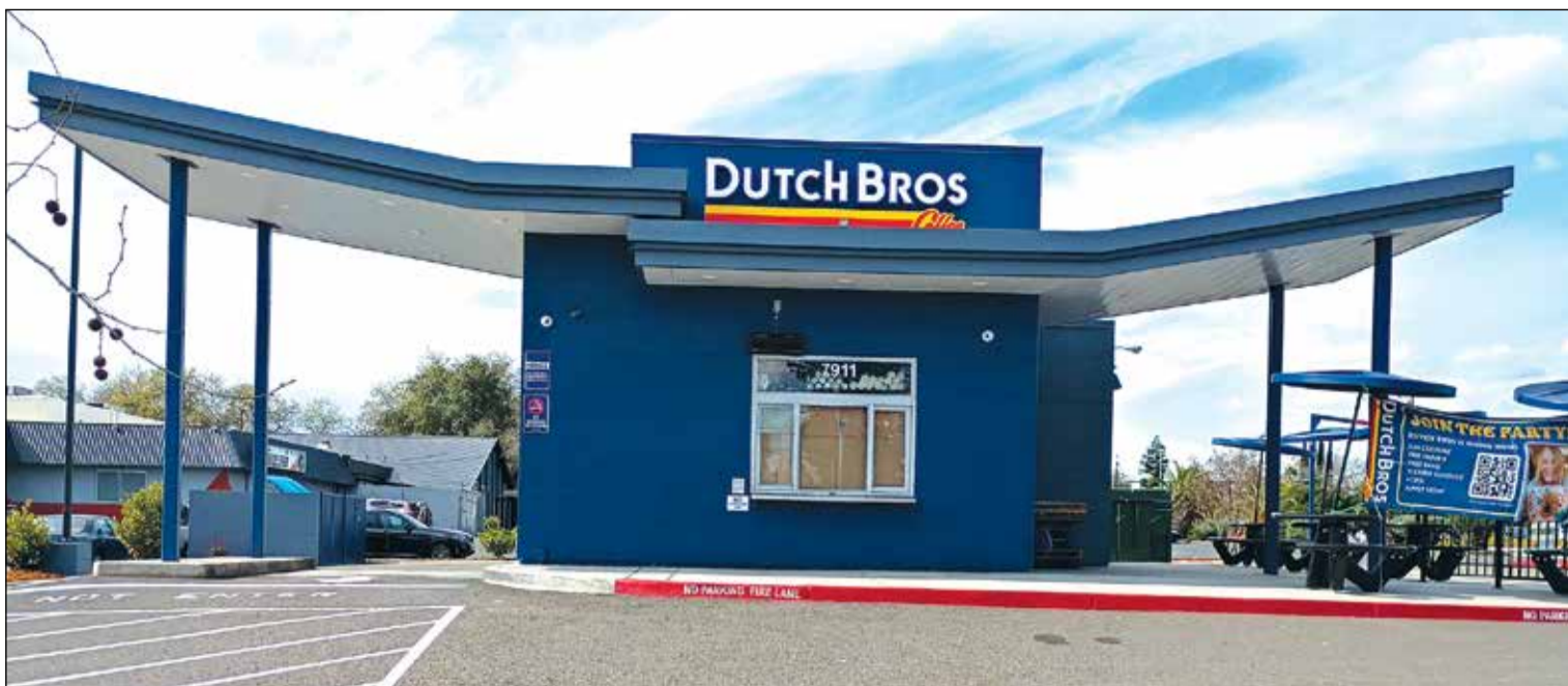
Construction work to convert a shuttered former Rally's Burger drive-thru at 7911 Auburn Blvd in Citrus Heights into a new Dutch Bros coffee shop is nearing completion.
