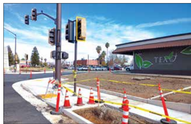
Construction on Auburn Boulevard has impacted business for Aquarium Depot, owned by Jason and Jeff Liang as well as for Just Tea It, a boba and tea shop owned by Jack and Amy Liang. Photo by Thomas J. Sullivan.
