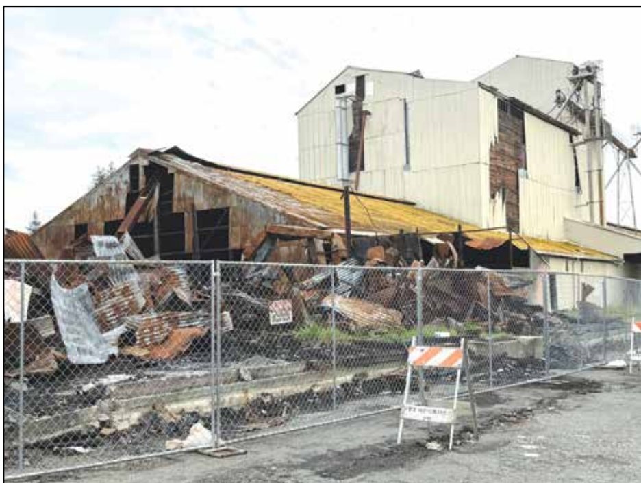
A newly installed fence secures the gnarled remains of the abandoned rice dryer at 110 Virginia St., now under the control of a court ordered receiver.
