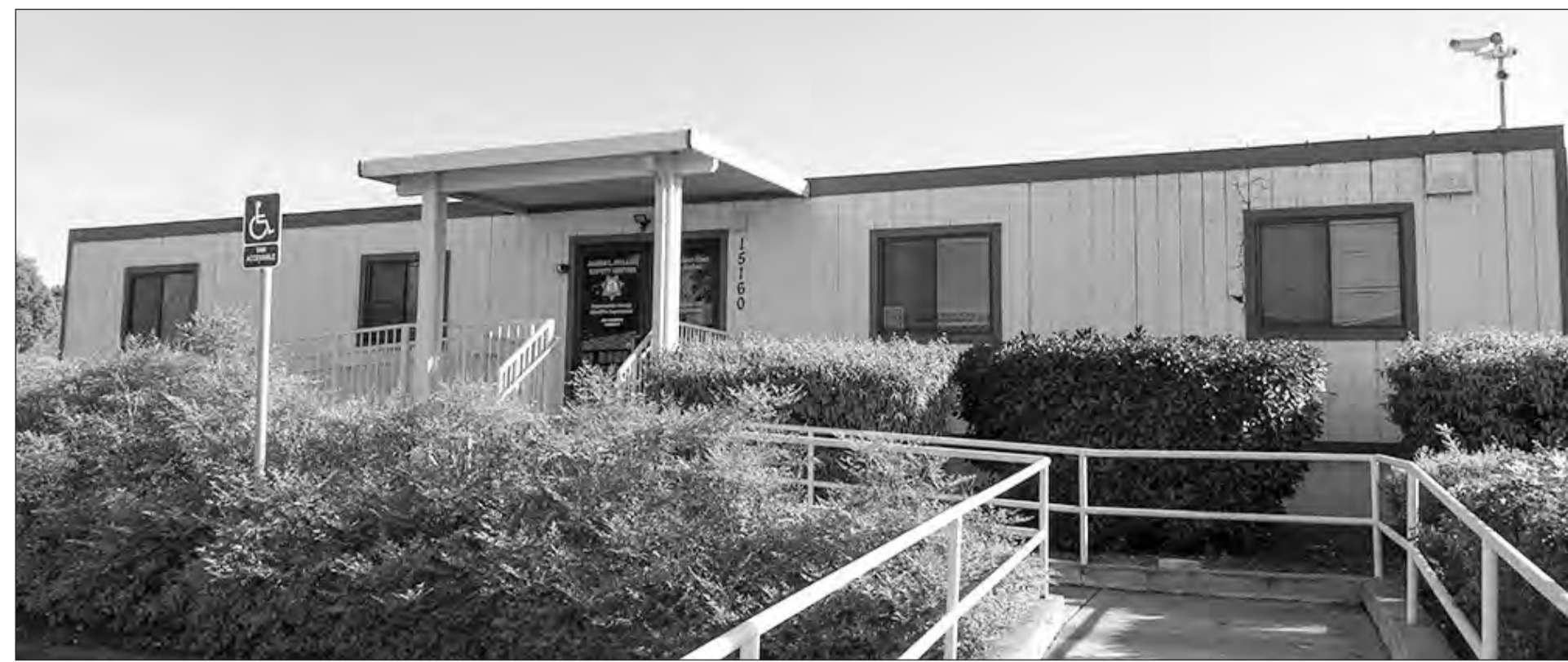
The Rancho Murieta Community Services District Improvements Committee recommends demolition of the district's deteriorating safety center, located across from the district office. File photo
