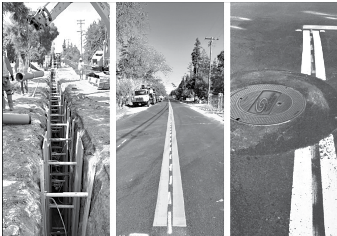
SacSewer connected homes to the public sewer system with newly constructed sewer pipes and manholes, and private septic tanks were safely decommissioned. Photo courtesy of Sacramento Area Sewer District
