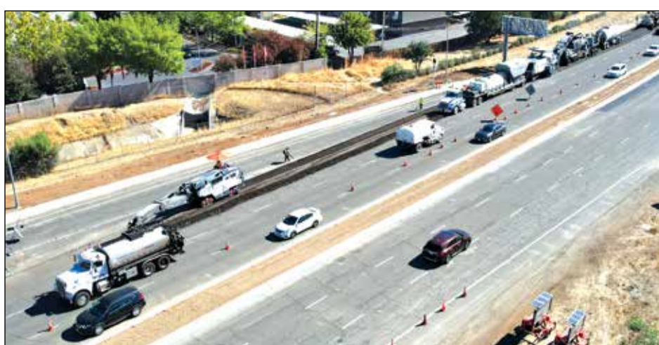
From major corridors to neighborhood streets, the Rancho Cordova Public Works team is hard at work upgrading roads across the city. Photo courtesy of the City of Rancho Cordova
