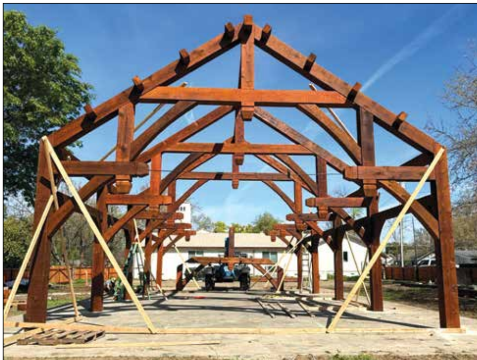
The redwood pavilion began drawing attention in the community as the timber frame rose earlier this month. This photo shows the initial placement of the structure before the beams were fully secured. Photo by Seti Long
