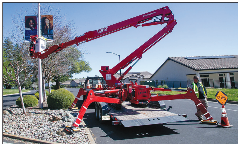
Daniel Esquivel directs traffic while a co-worker installs senior banners from the association's new aerial lift along Murieta Parkway.
