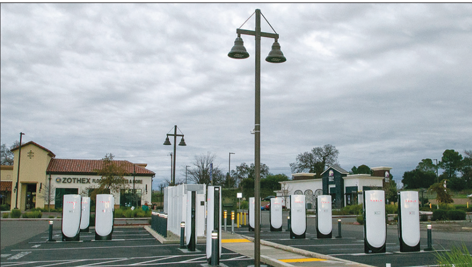
The Tesla Supercharger station is now operating in the Bel Air Market parking lot.
