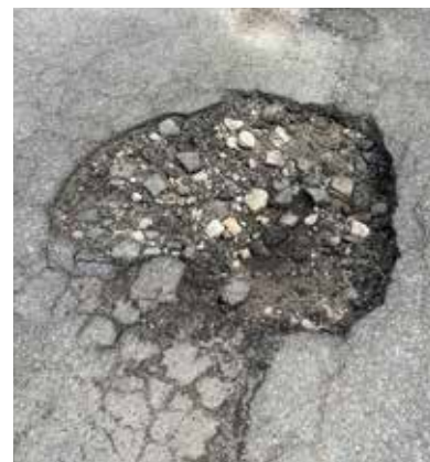
Potholes are ugly and can cause serious vehicle damage.
