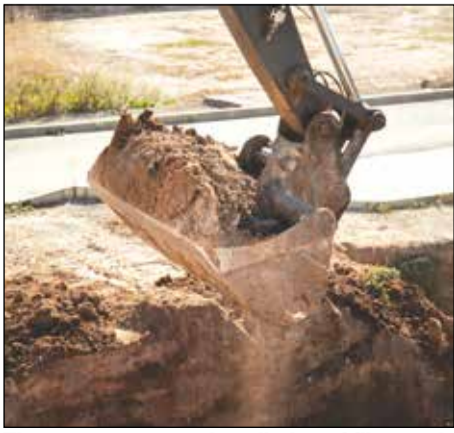
The program covers installation of fiber optic infrastructure, including underground conduit up to 12 feet deep and utility poles up to 150 feet high. Image by Freepik
