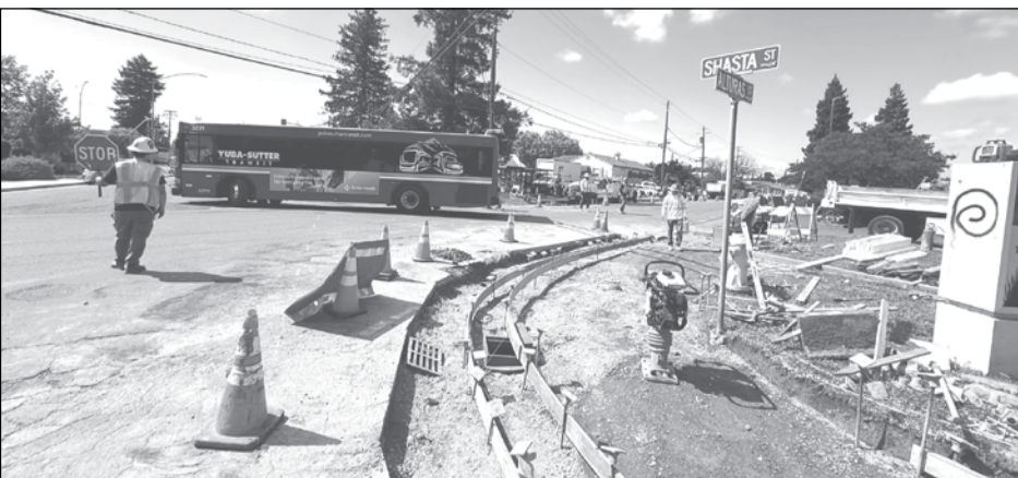
Construction crews work on roadway and pedestrian improvements near the Yuba-Sutter Transit Authority bus stop at the corner of Shasta and Alturas streets in Yuba City. The project includes a new concrete bus pad, ADA upgrades, drainage repairs and roadway rehabilitation. Photo courtesy of the City of Yuba City
