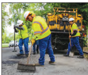
The city reported that 7,761 potholes were repaired in 49 days following a citywide effort to identify streets and intersections in need of repair. Photo courtesy of City of Sacramento
