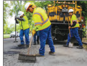
The city reported that 7,761 potholes were repaired following a citywide effort to identify streets in need of repair. Photo courtesy of City of Sacramento
