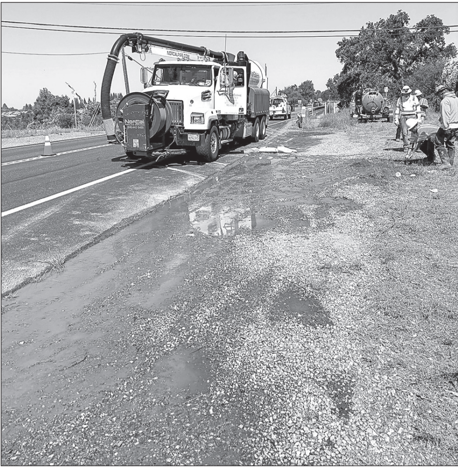
A sewage cleanup closes one lane on Jackson Highway east of the Yellow Bridge on May 17. Photos courtesy of Rancho Murieta Community Services District
