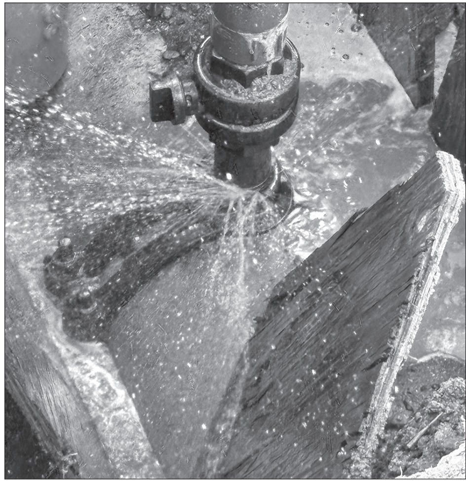
Sewage sprays from the corroded connection that failed.
