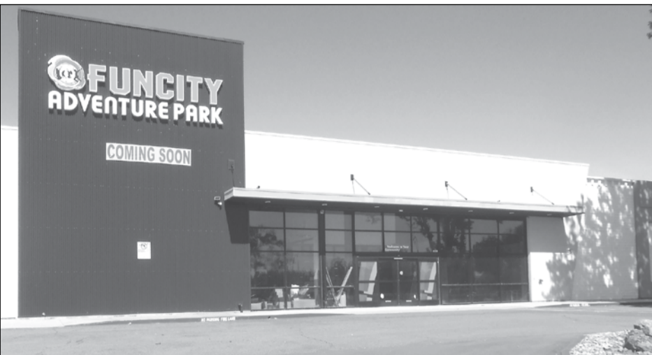
Several families and their children who stopped by to enjoy some morning summer fun on opening day were turned away by workers inside who continued to assemble arcade games and other equipment without available electrical power.
