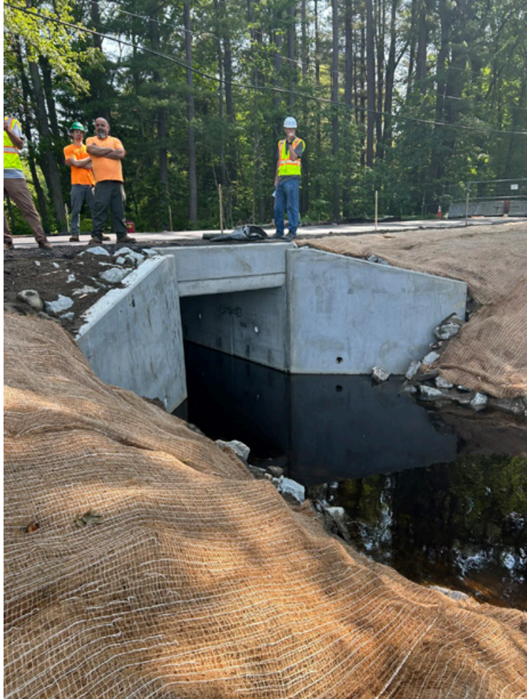
Schoolhouse after removal - culvert under 8 Lots Road. Photo supplied by Caleb Slater
