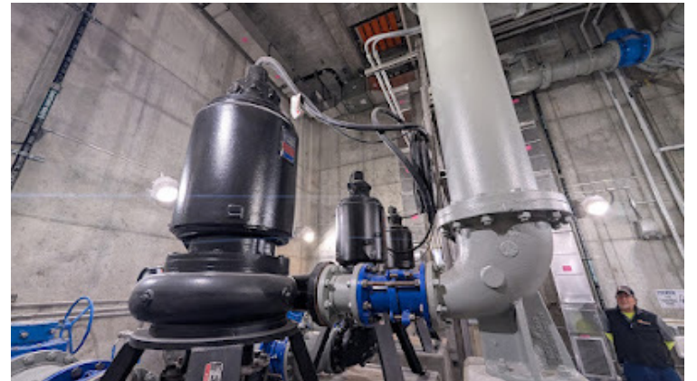
25' Underground and inside the new BSI Lift Station on Beaver St Photo by Franklin Matters
