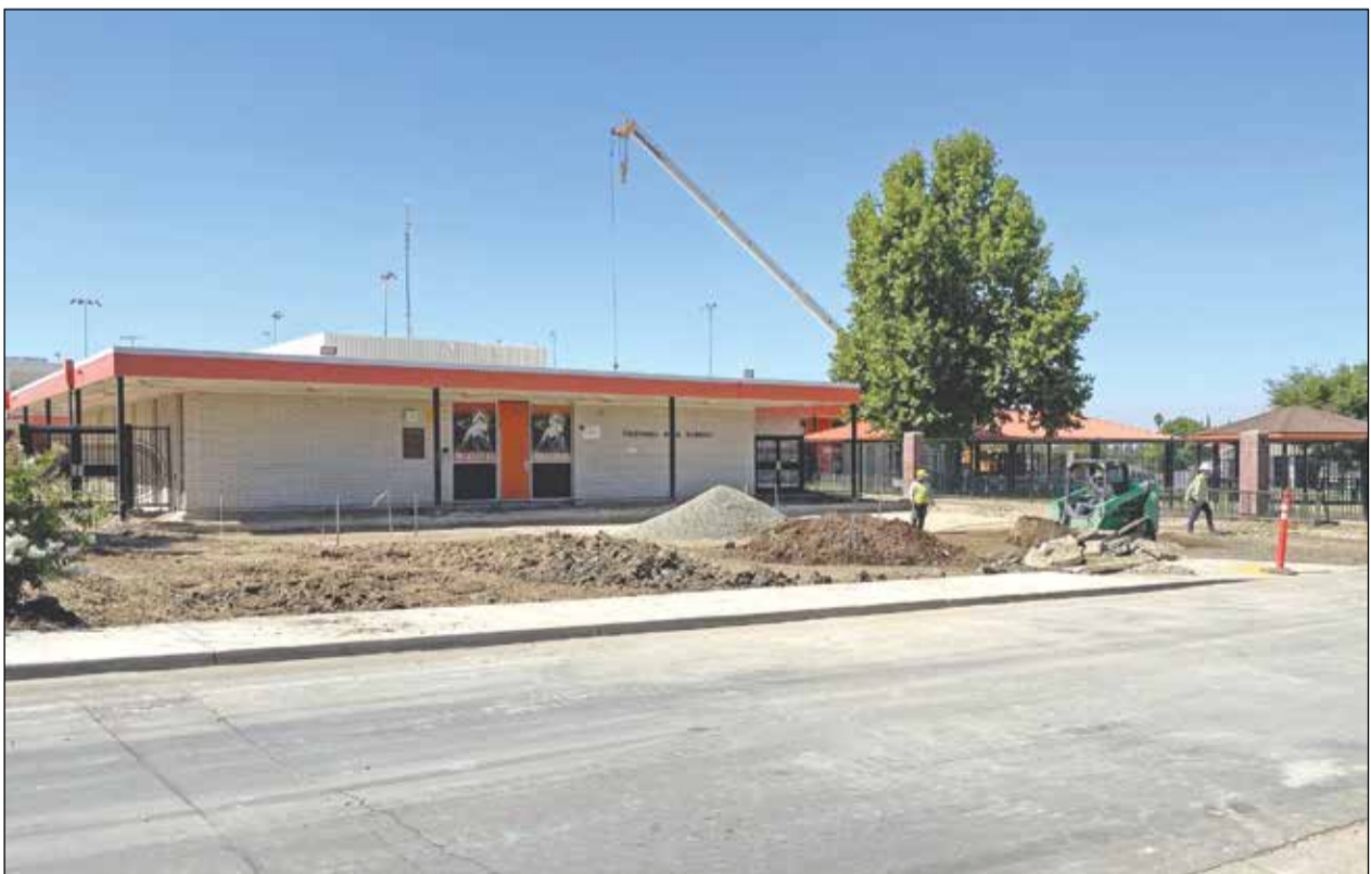
Schools across the Twin Rivers Unified School District are undergoing construction projects during the district's summer break. Photo courtesy of Twin Rivers Unified School District
