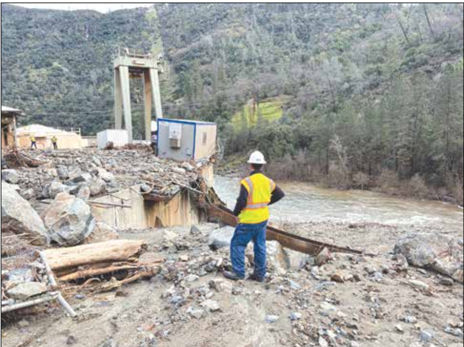
A small team recently made initial site visits to Yuba Water’s New Colgate Powerhouse in Dobbins to survey damage and begin work to establish safe access to the powerhouse facility following the Feb. 13 penstock rupture on the hillside above. Photo courtesy of Yuba Water Agency
