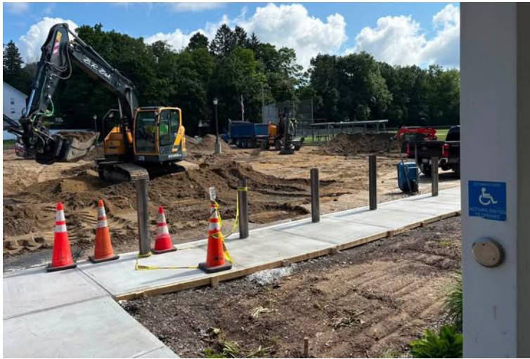
View of the parking lot from the Holden Senior Center.
