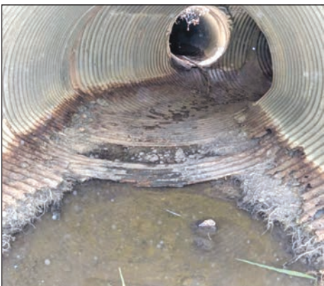
Image shows a damaged culvert under Pera Drive. Photo courtesy of Rancho Murieta Community Services District
