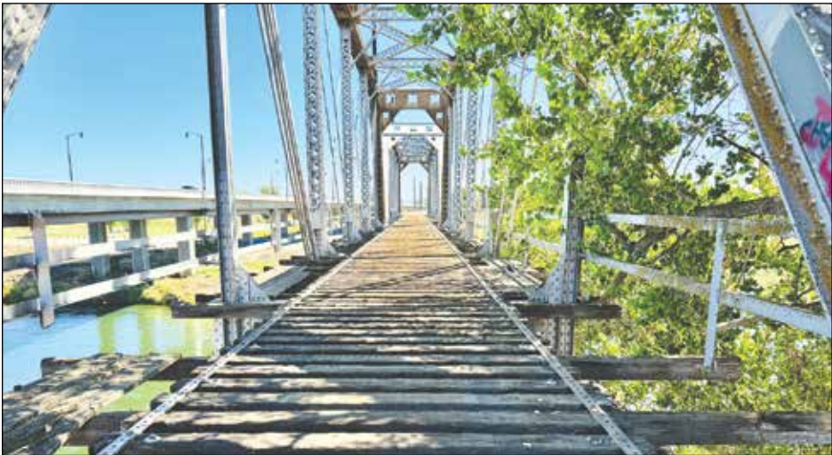
The old railroad trestle runs alongside the Fifth Street Bridge between Marysville and Yuba City. No gates, chains or warning signs were visible at the approach when the Territorial Dispatch visited the site Aug. 16.
