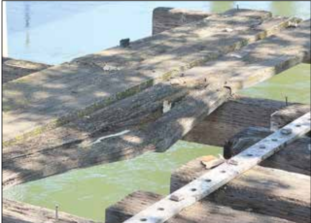
Deteriorated wooden ties and open gaps are visible along the old railroad trestle beside the Fifth Street Bridge between Marysville and Yuba City. The structure has come under scrutiny following the Aug. 9 death of a 13-year-old girl who fell from the trestle.
