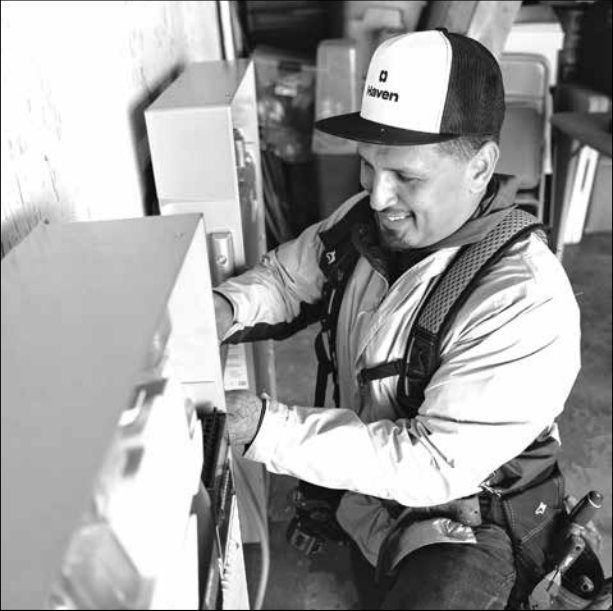
Available to customers of participating publicly owned utilities, the program can cover the cost of a home battery system, as well as solar, and includes installation. Photos courtesy of Haven Energy
