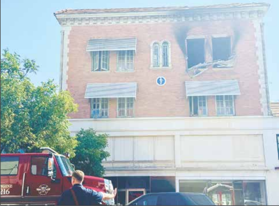
Fire damage is visible around the upper-floor windows of the 423 Apartments in downtown Marysville on Sept. 11, the morning after a fire heavily damaged part of the D Street building.
