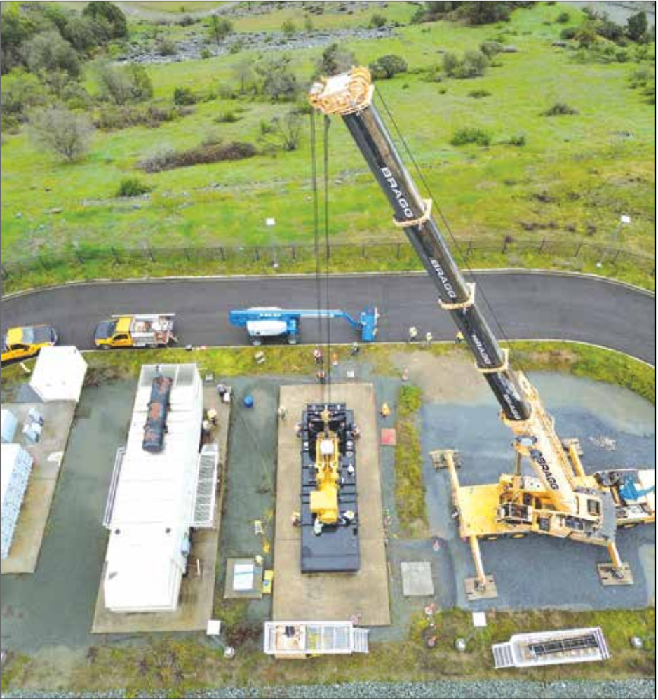
Standby power at PCWA pump stations is one of the projects included in the Water Connection Charge update and will help support delivery of American River water to the future Ophir Water Treatment Plant. Photo by Joel Schaap/PCWA
