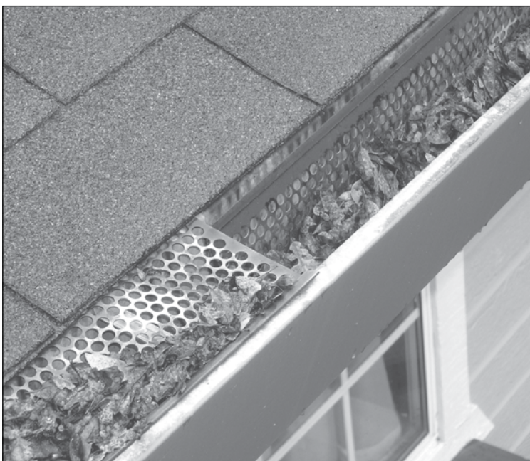
Review your emergency plan and supplies, including clearing leaves and debris from gutters, drainage areas and storm drains around your home. Photo by 123switch via Pixabay
