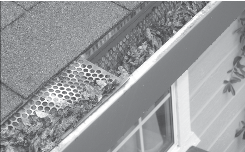
Review your emergency plan and supplies, including clearing leaves and debris from gutters, drainage areas and storm drains around your home. Photo by 123switch via Pixabay
