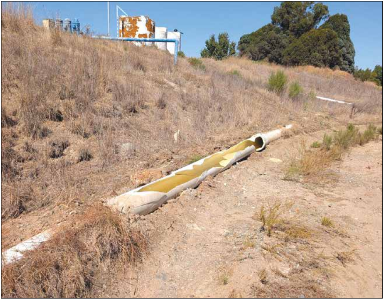
Photo shows the damage to a spray field main that has since been repaired. Photo courtesy of Rancho Murieta Community Services District
