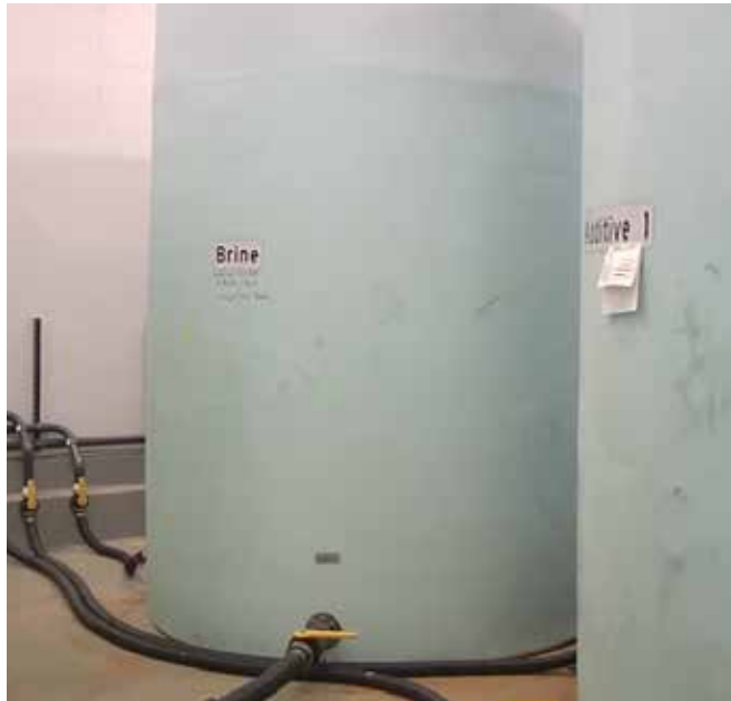
Brine and chemical storage tanks at the Maple Grove Truck Station
