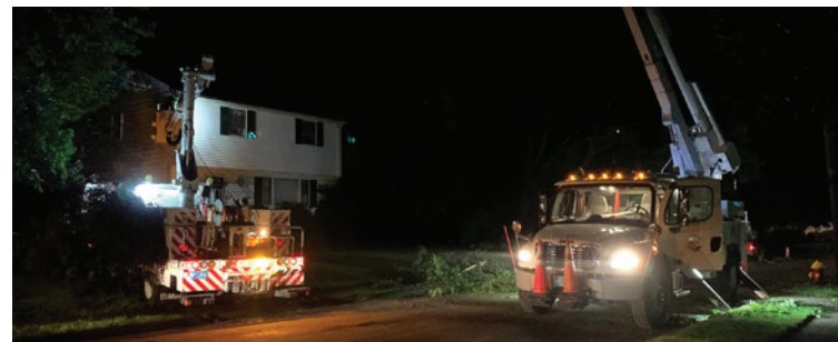
Norwood Light crews responded to multiple outages, including a broken primary cable on George F. Willett Pkwy, downed limbs on Jacobsen Dr & a damaged switch at Walpole Street and Geraldine Drive. A view from the Norwood Police/Fire Station on Nahatan St.
