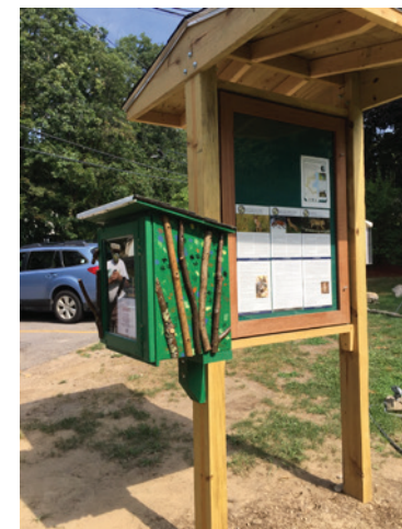
Mike Jones built the library at the new Oak Street entrance to the town forest. (Photo/supplied)
