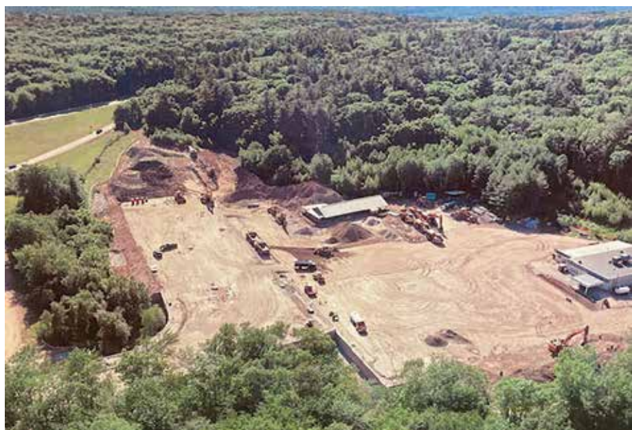
An aerial view of the former Serendipity grounds on Douglas St. in Uxbridge, where Amazon will set up a sortation facility—a deal transacted by GBI Avis' Tracy Sharkey.
