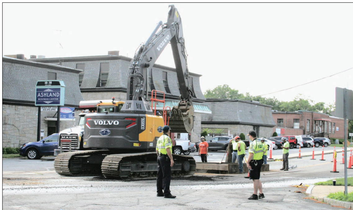
Road Construction Continues Crews continue construction work on the Route 126/Pond Street Revitalization Project and on the Downtown Revitalization Project on Main Street and Front streets. This work is significantly impacting traffic. Please plan your travel accordingly. For updates and to sign up for a direct email newsletter, visit ashlandmass.com/160/Department-of-Public-Works . (Photo/Cliff Wilson)
