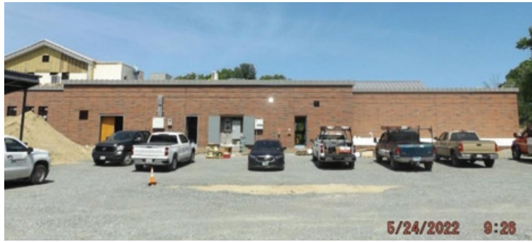
The Progress of the exterior at the rear of the fire department side. Photos courtesy of the Ashland Public Safety Building Facebook page
