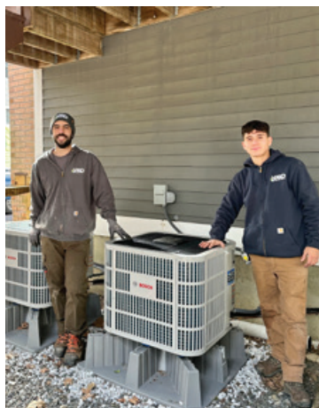
The professionals at Pro Comfort Control bring their expertise in heat pumps and all facets of heating and cooling systems to the Holliston community.
